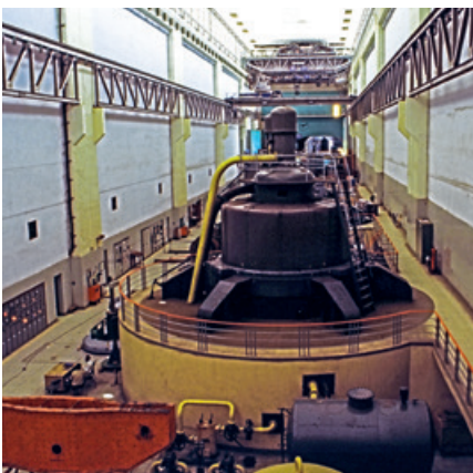
The turbines of the Aswan Dam
